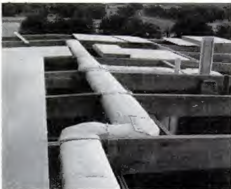
Solid-core panels make up the roof deck. This construction view shows the insulated air-conditioning duct that extends along the center hall. Entire house was erected in two weeks
